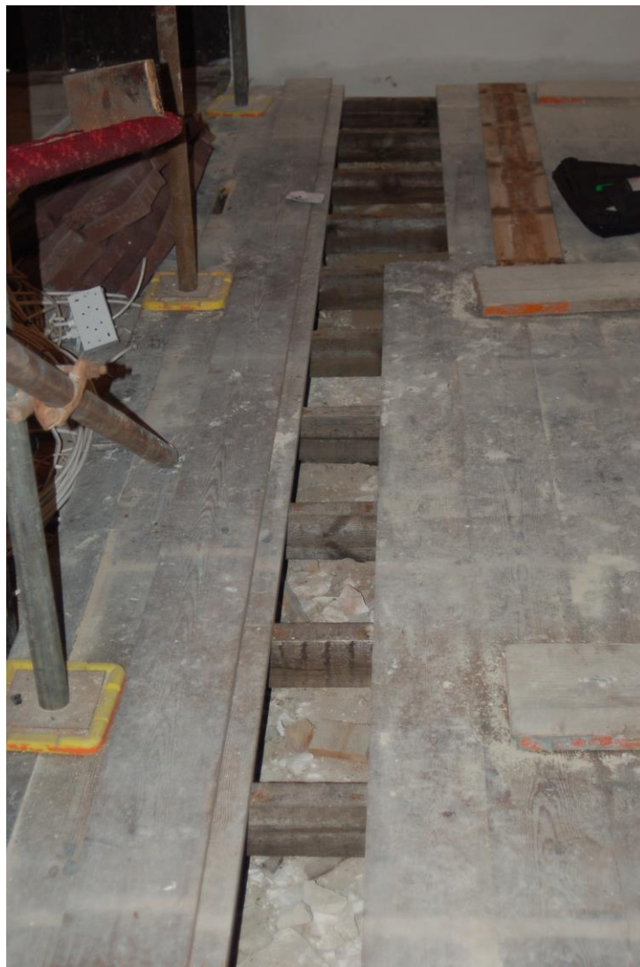
Suspended Victorian wooden floor revealing a void below at the Grade I listed, 12th-century, Church of St Mary, Maiden Newton. Image reproduced by kind permission of Steve Wallis, Dorset Council.
